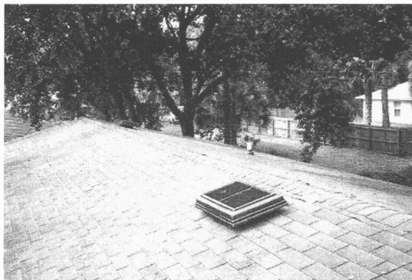
Figure 2. Photo of PV ventilators.
